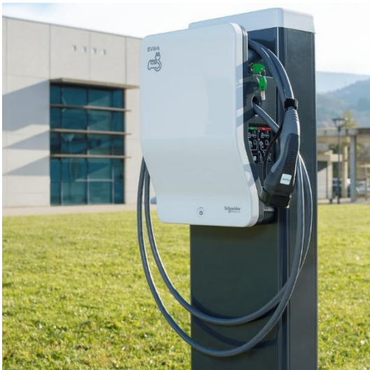
Figure 7 EV charging system example.
